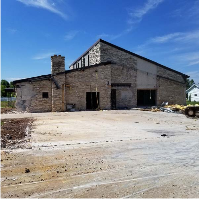
Image #10: Standing in the old fellowship hall looking at the north wall of the church
