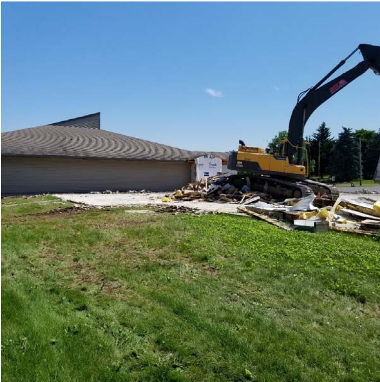
Image #8: Excavator is sitting in the old fellowship hall. Removal of the last couple of loads of debris from that area is in progress
