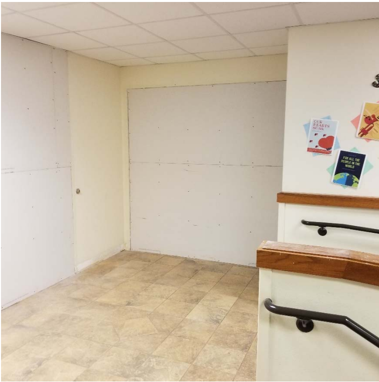
Image #1: Existing door opening at top of ramp has been studded shut.
