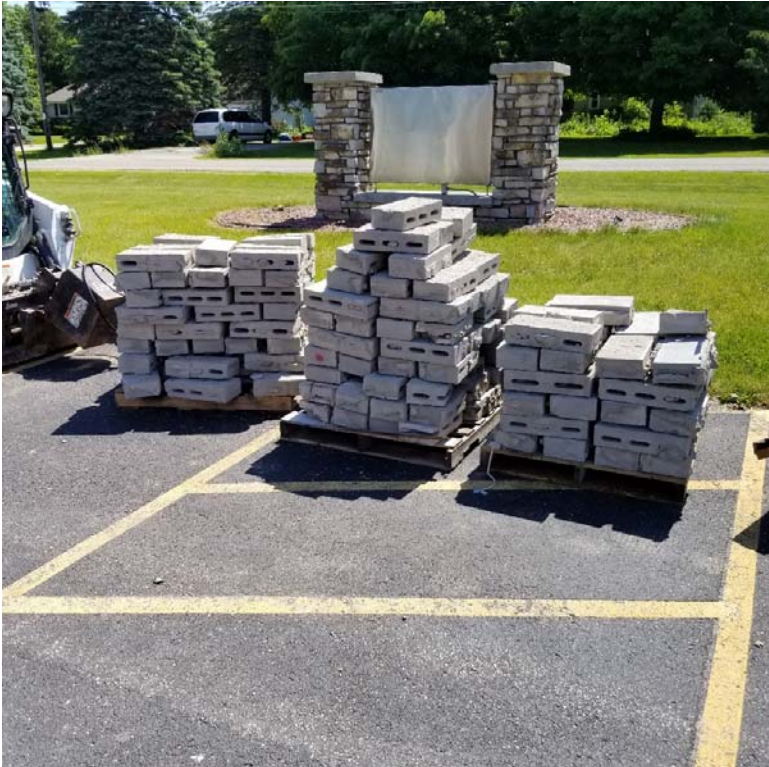
Image #12: Existing split face masonry has been salvaged and stored (per drawings) so that it can be reused as infill at new connecting corridor
