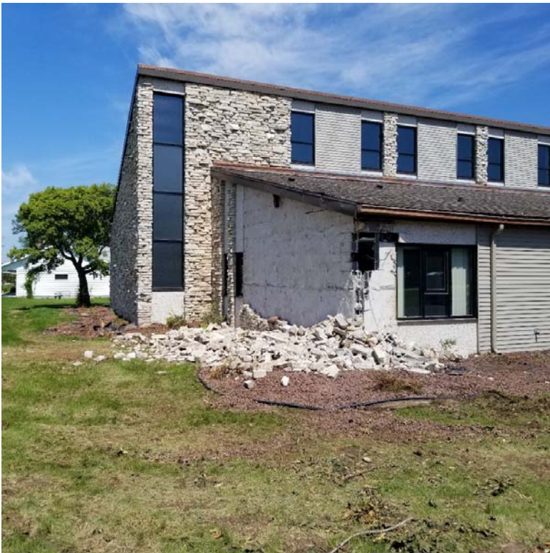
Image #4: Southeast corner of the church. Stone has been peeled off and will be stored on-site for congregation members to use.
