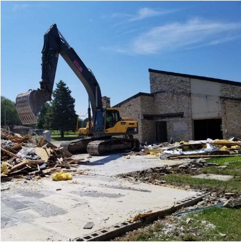
Image #9: Excavator is sitting in the old fellowship hall. Removal of the last couple of loads of debris from that area is in progress
