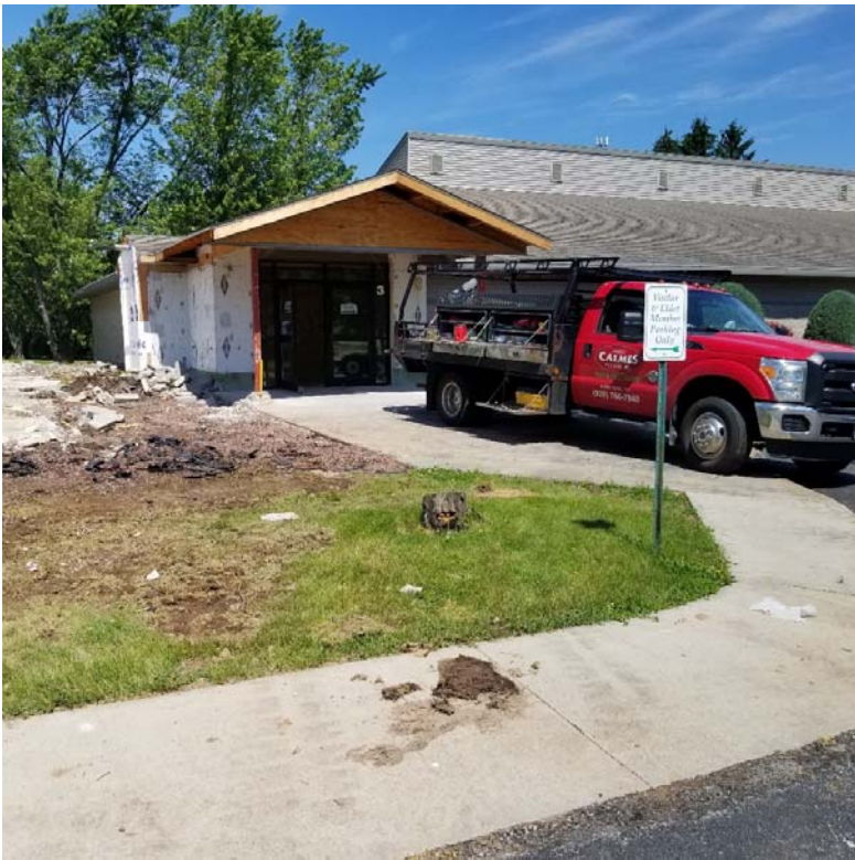
Image #11: Demolition of the existing entry to the church offices has begun.
