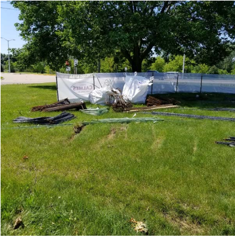
Image #3: Re-bar is being stored on south end of site. This should be on wood blocking above grade to avoid rusting
