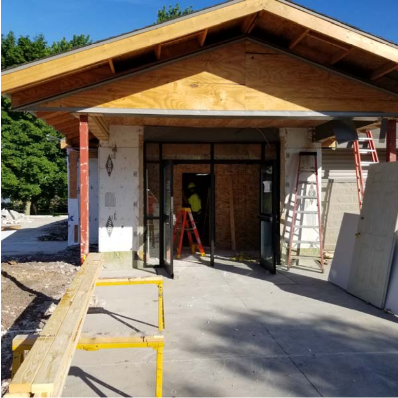
Image #1: New (temporary) egress door is being cut/framed into the east wall at the top of the ramp.
