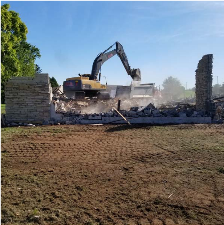
Image #7: Only the south corners of the church remain in place.
