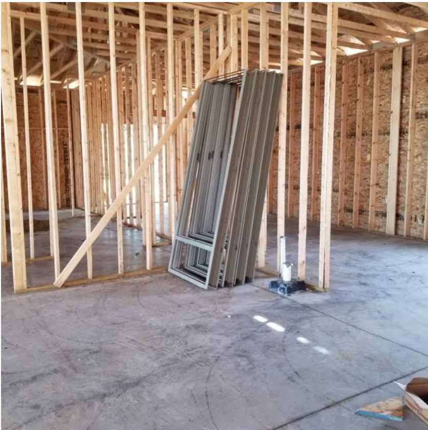
Image #5: Hollow metal frames are stored directly on concrete- they should have wood blocking under them to avoid rusting.
