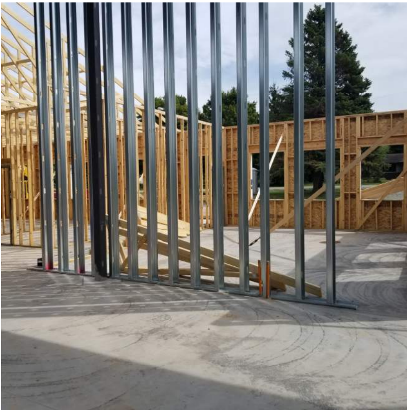
Image #8: Steel stud wall between green room and sanctuary. Need to cut a door opening in this wall per owner request.
